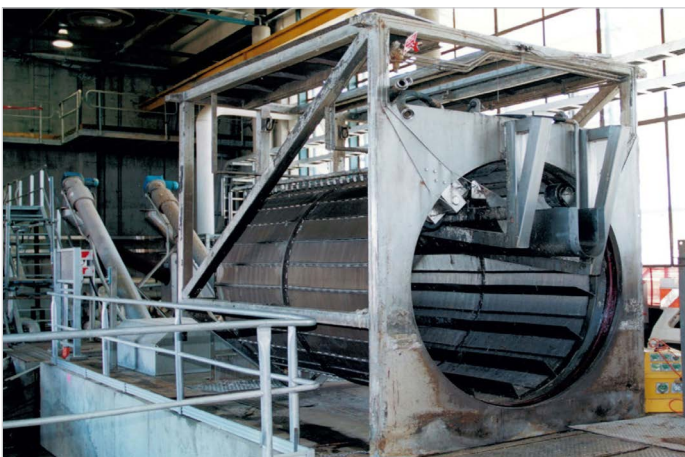
A view of one of the stainless steel fine screens prior to installation.
